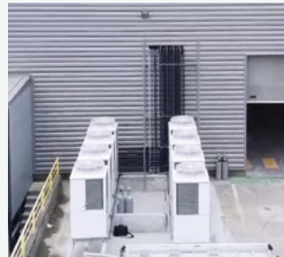
STEMCELL Technologies, a global biotechnology company, installed CO 2 condensing units - CR Series for cold rooms in the warehouse. France. Refrigeration
